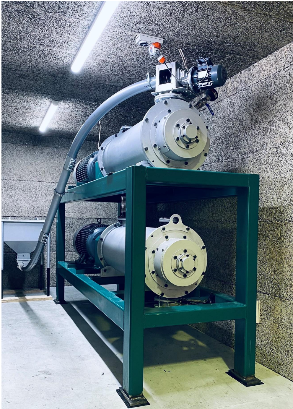
Dual cascading reactors reduce / transform mussel shells into calcium carbonate.
